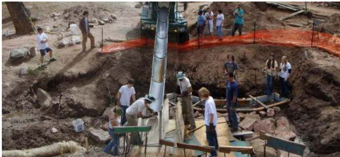
Manitou Springs HS Students pouring bridge footings under the direction of CC staff.
